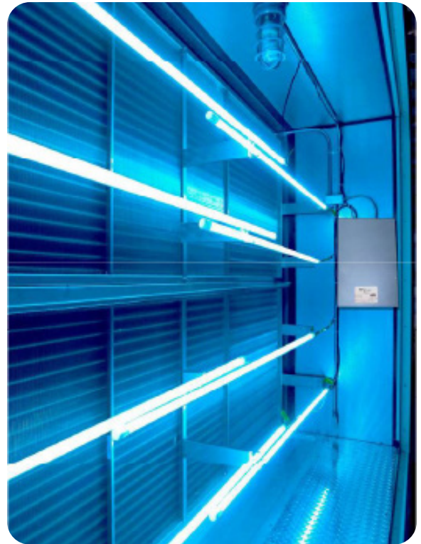
The market-leading RLM Xtreme™ UV-C lamp system from UV Resources is one of the most effective germicidal HVAC solutions available today.
